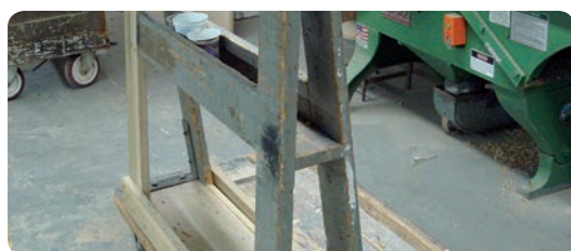
Wood - Splinters and rots
